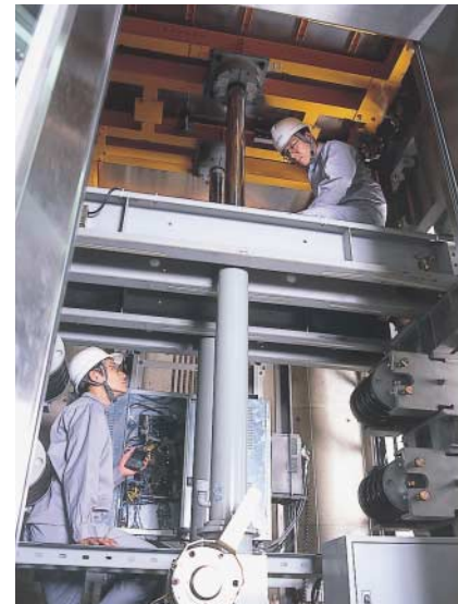
Development of the double-deck elevator
