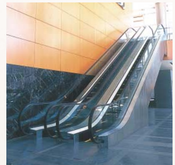
A Fujitec escalator installed at the Bank of Boston Headquarters Building in Buenos Aires
