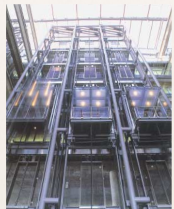
Elevators operating at the HaLo Building in Chicago
