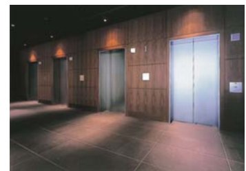
Fujitec elevators working at Roppongi Hills Gate Tower in Tokyo
