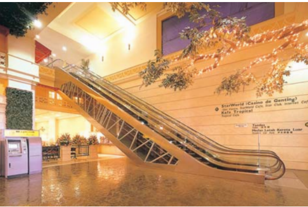
Fujitec escalators working at the First World Hotel in Malaysia
